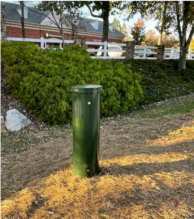
Figure 4: Cylindrical ground furniture can place support electronics up to 20 feet away from a pole with mounted 4G/5G radios.
