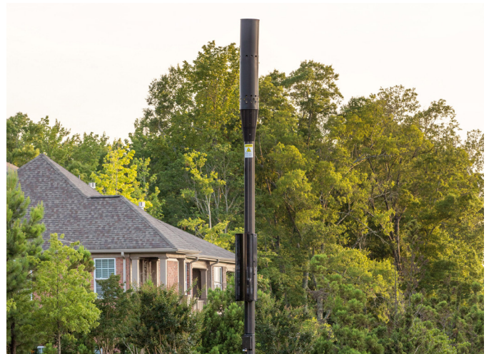
Figure 1: Streetlight poles are an obvious option for urban small cells, and the top of the pole provides the best line of sight for 5G coverage.
