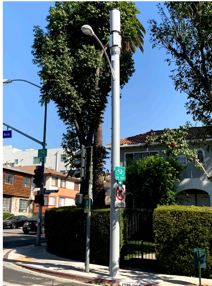
Figure 3 - 5G Small Cell light pole for the City of Los Angeles Bureau of Street Lighting
