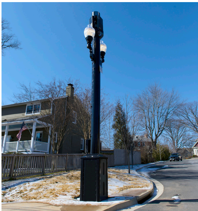
Figure 2 - Installed Small Cell light pole in Arlington County
