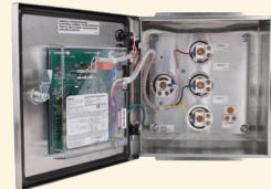
Three Phase Wye SPD with four Strikesorb 40s in an optional stainless steel enclosure with alarm.
