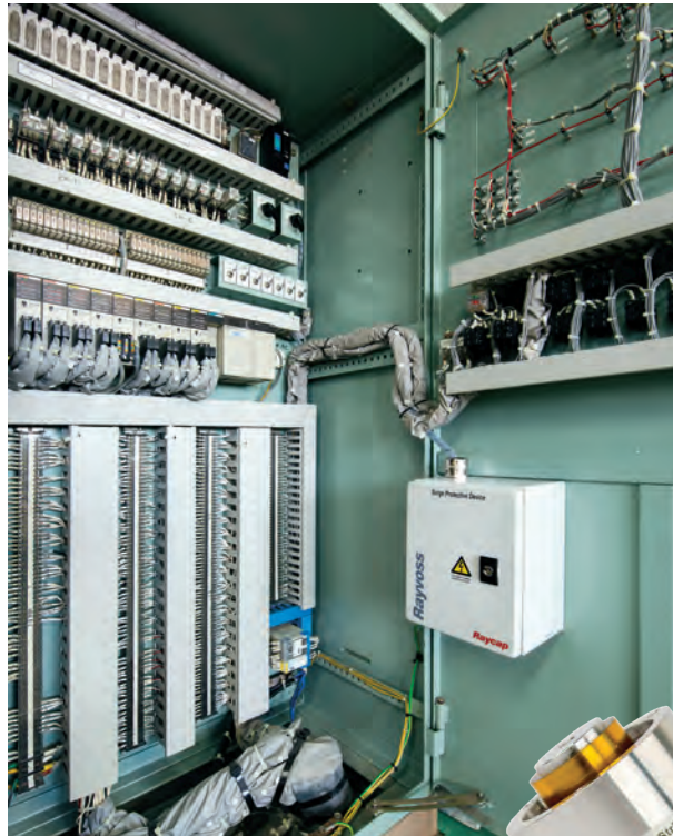
Figure 2: Rayvoss M surge protective device installation on the inert gas control panel.
