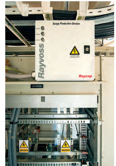
Figure 3: Rayvoss M systems strategically placed at the Emergency Switch Board (ESB) of the vessel provides vital protection to critical shipboard functions.
