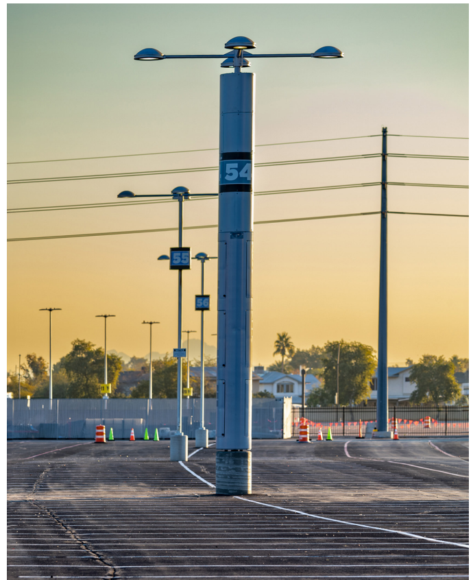
Figure 2. Raycap's expertise made it the best choice for this concealed small cell pole project, overcoming a tight schedule, complex thermal designs, incorporation of existing light arrays, and designing a new multi-carrier AC disconnect.
